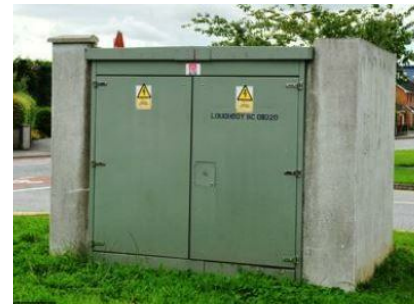
SAMPLE IMAGE OF TYPICAL UNIT STANDALONE SUB TO ESB SPECIFICATIONS APPLIES TO ALL SUB STATIONS
