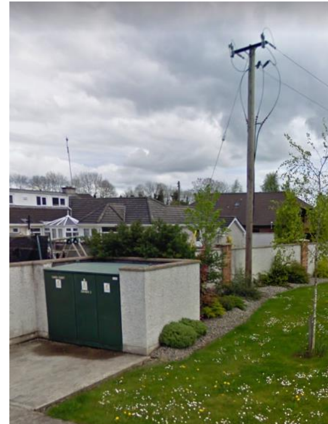
Existing Sub Station and Pole at Cairn Court
